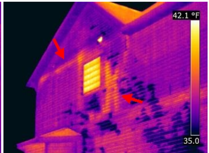
Indication of air leakage at the ceiling/wall of the second-floor left rear bedroom. Also air leakage is evident adjacent to the window from floor to ceiling.
