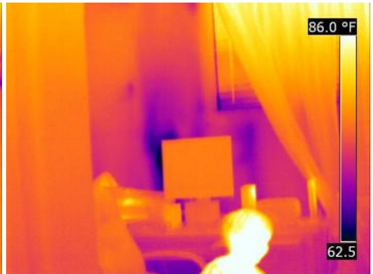
Air infiltration through the wall behind the office desk/computer screen.
