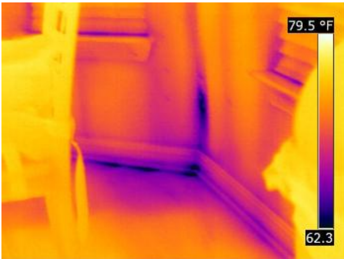
Air infiltration in the kitchen dining area at the electrical outlet and below the baseboard from a leaking wall framing plate.
