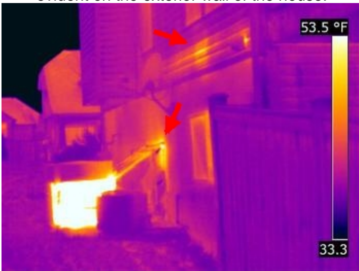
Indication of air duct leakage at the unit and through the first floor wall. Note that there is air leakage along the entire rim joists just above the foundation.
