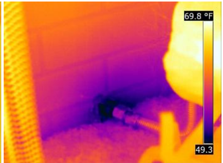
Indication of air leakage into the wood fabricated chimney/fireplace appliance. Interior infiltration has been sealed but external infiltration of the wall system is still occurring and there is likely insufficient insulation installed.
