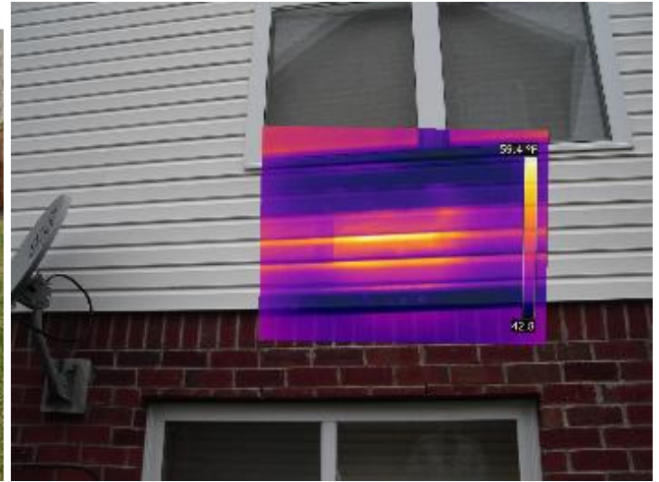
Indication of a leaking air duct from the interior of the house. Air is leaking between the basement ceiling and first floor.
