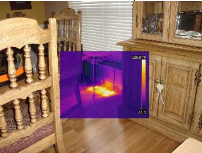
Indication of air loss at the supply air boot below the register.
