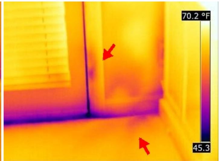
Air infiltration at the basement entry door as well as areas behind the office desk which is indicating considerable air infiltration from behind the desk.
