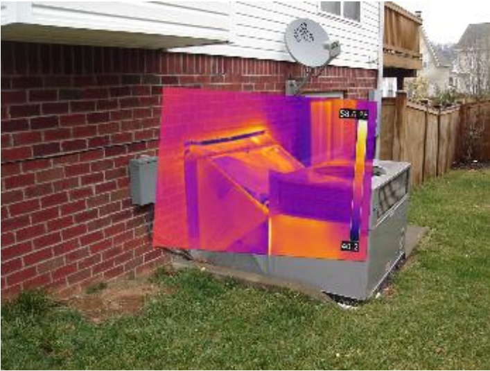
There is an apparent leaking air duct at the outdoor HVAC system. This will produce a considerable efficiency loss.
