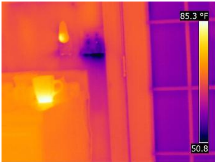
Air infiltration through the light switch at the rear kitchen entry door.
