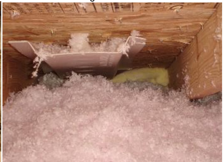
There is still indication of heat loss at the junction of the ceiling and wall in the left rear second-floor bedroom. Air leakage past the installed insulation and insufficient insulation at the eve is likely creating this heat loss.
